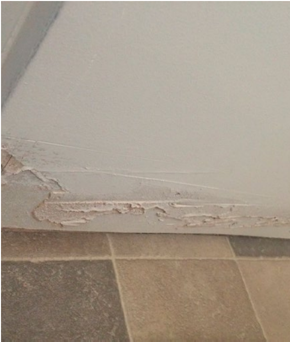
Look for chips or scrapes in plaster on walls, or bumps where it's been filled and not sanded down.
